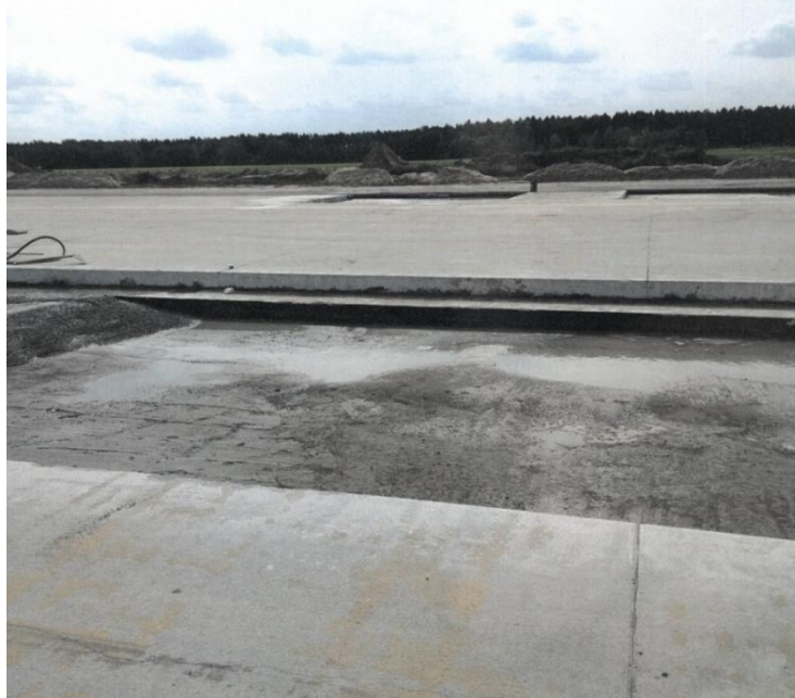
5. There is a layer of water in the place where the concrete mix is to be placed
