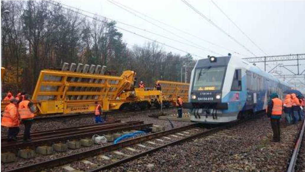
4. Delivery to the construction site ordinary crossings using the platform of "Switcher"
