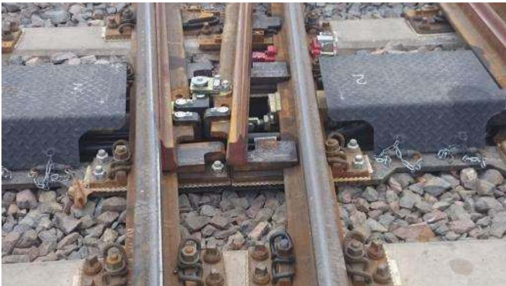
12. Fragment of fastening elements closing adjustment Spherolock in the switcher complex switch Rkpd 60E1-190-1 :9 from Vossloh Cogifer Poland Sp. z o.o
