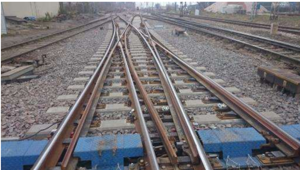
8. The crossover switch of Track Tec KolTram Sp. z o.o visible rolls underspires "Austrollor"
