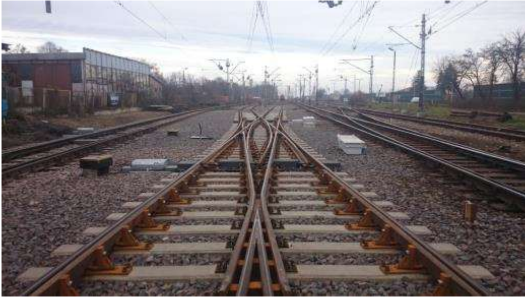
11. View of of the overbuilt switch Rkpd 60E1-190-1 :9 from Vossloh Cogifer Poland Sp. z o.o on Swidnik station as a switch 24
