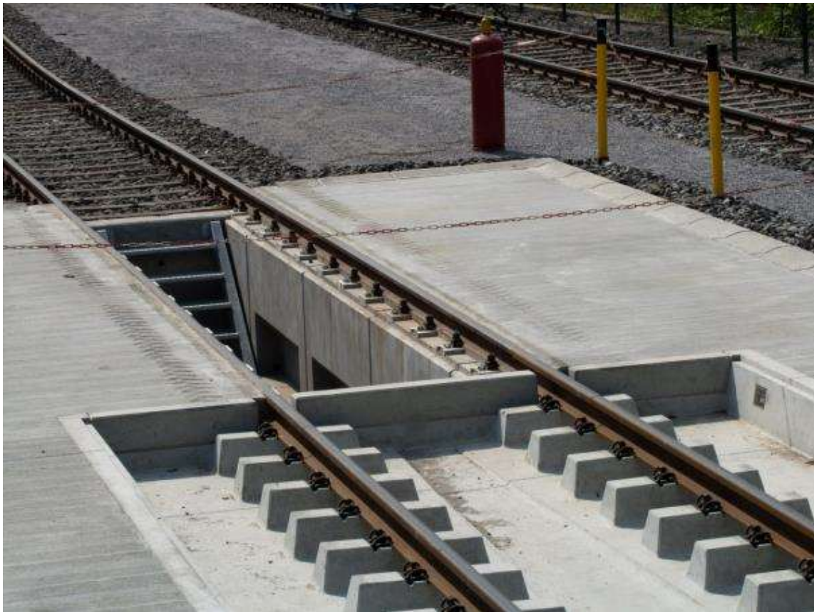
3. An example of the point of rolling stock maintenance - channel inspection of AG system and bath-track GTW system (Pic. BFL Lauchhammer)
