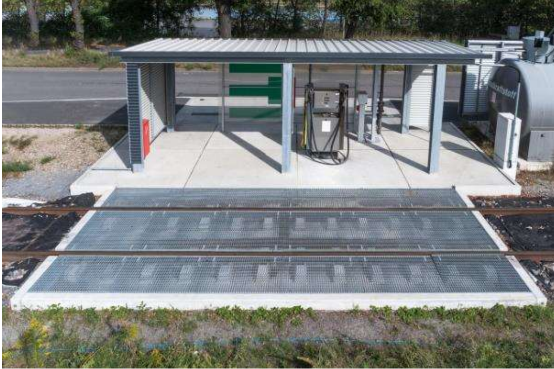
4. Eco-friendly fuel station for refueling locomotives, made of non-ballasted reinforced concrete precast system GTW
