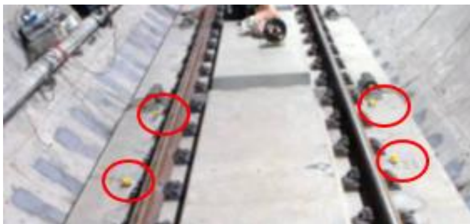
11. Location of measuring sensors on a concrete slab with a spring vibration isolation system on the metro line No. 10 in Shanghai.
