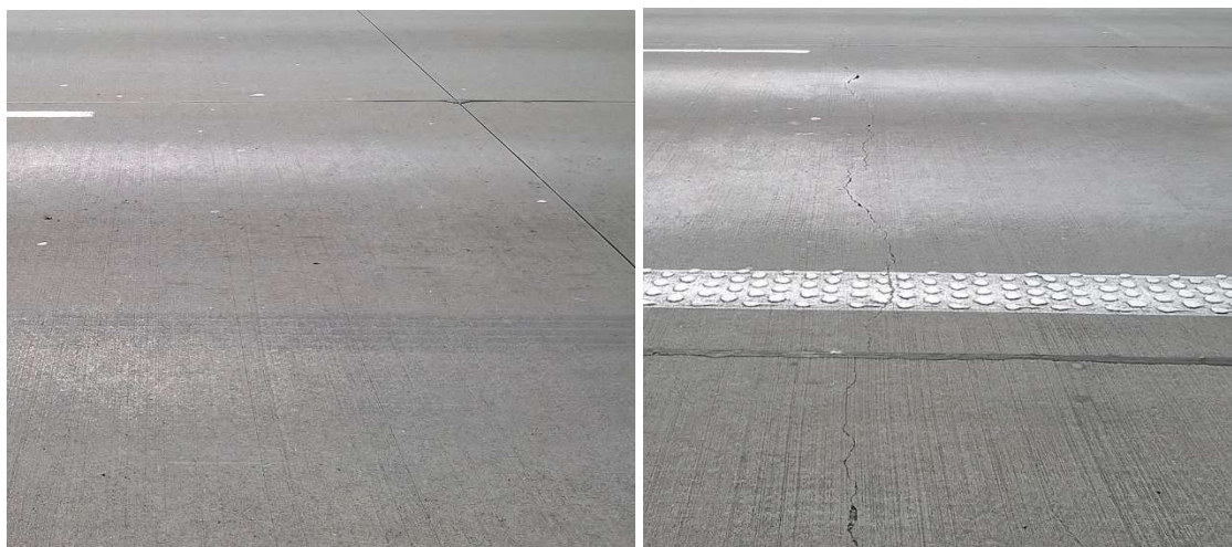
3. The A4 motorway - paved surface (left) and continuous reinforcement (on the right)
