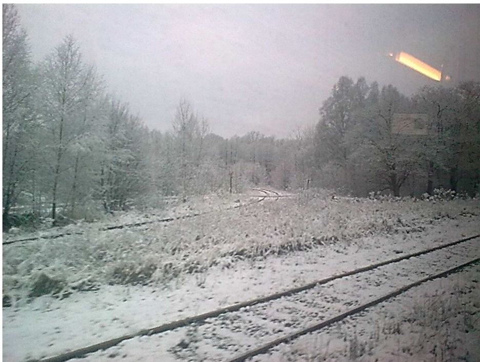
9. View of the departure of the siding to the plants of Nowy Łąd sp. O.o. Gypsum and Anhydrite Mine in Niwnice
