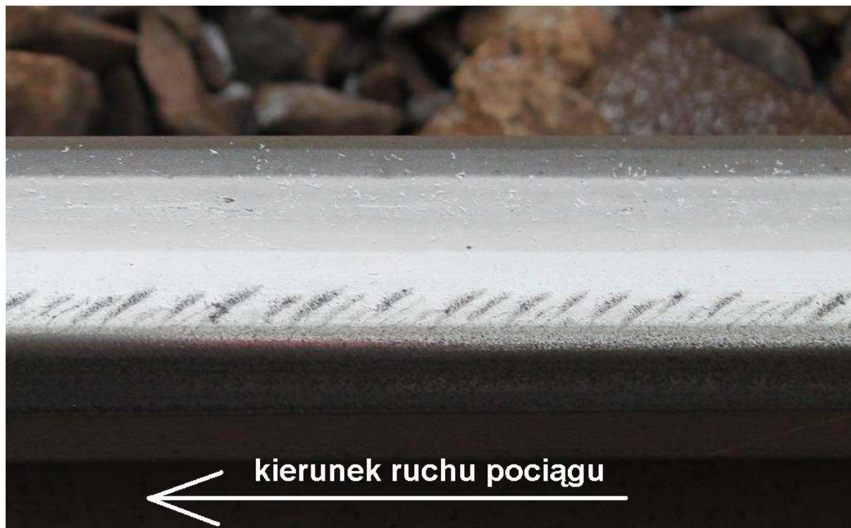
1. An example of a headcheck defect
