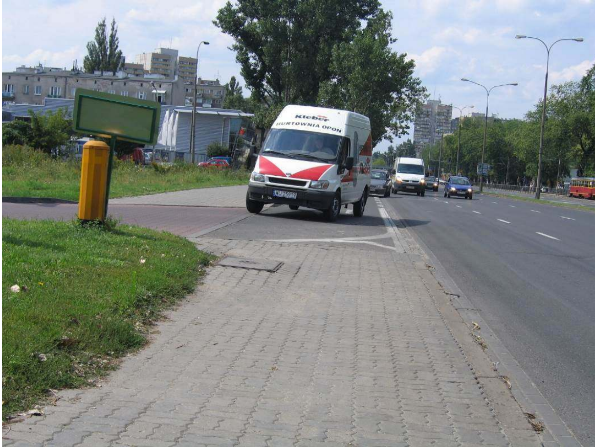
13. Improperly performed correction of the pavement course poses a threat to the movement of visually impaired and blind people - Warsaw/Poland
