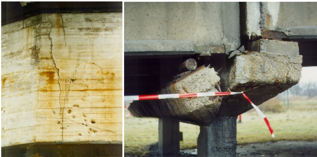
13. Loss of material continuity: scratches (left) and fracture (right)
