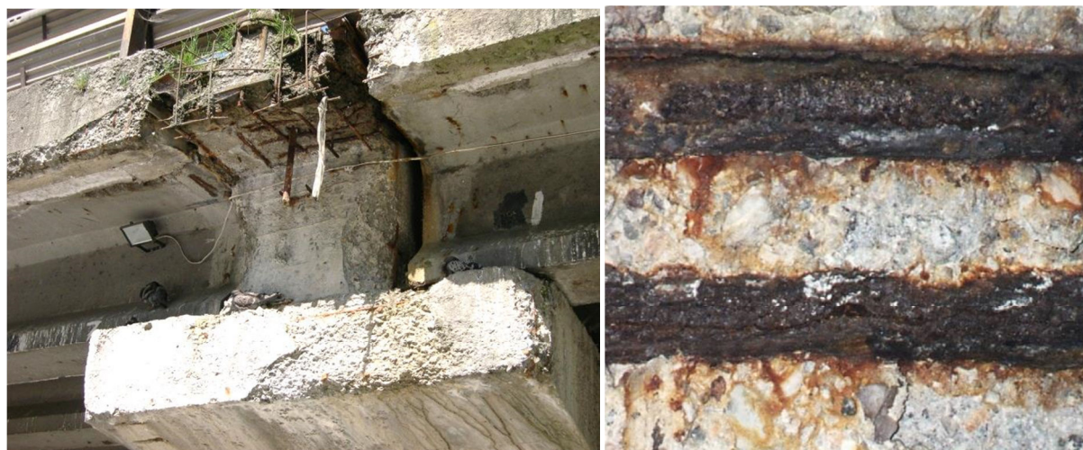
11. Destruction of concrete and steel of reinforcement bars in the form of deterioration of chemical and physical properties of materials - occurring simultaneously with material losses
