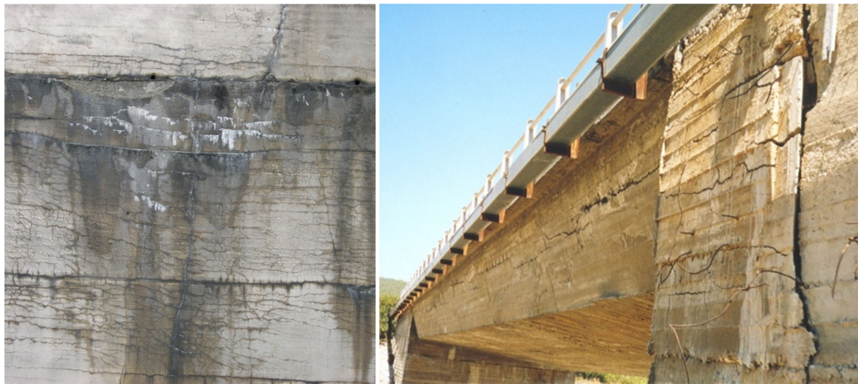
7. Examples of the destructive material degradation effects : concrete scratches and destruction caused by cyclic freezing/thawing of water and washing out of concrete components (left) and concrete shrinkage (right)
