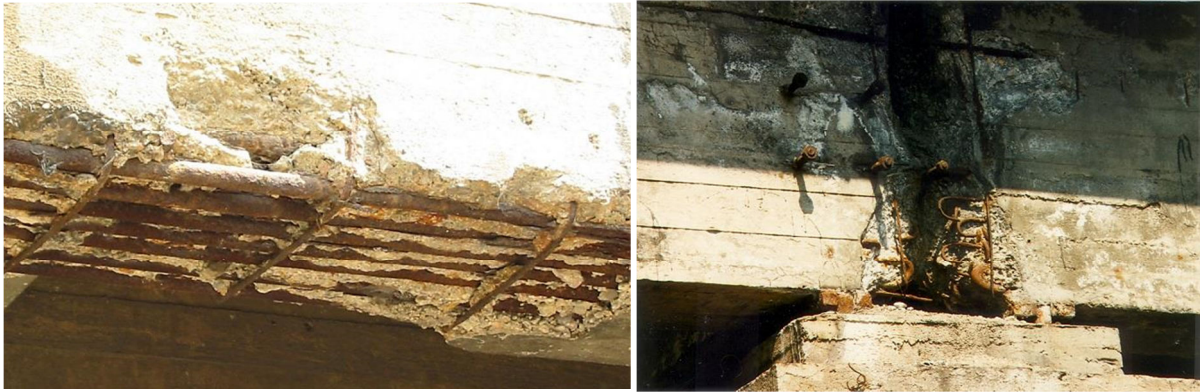
12. Loss of concrete in the protective layers and losses of reinforcing steel in bridge girders
