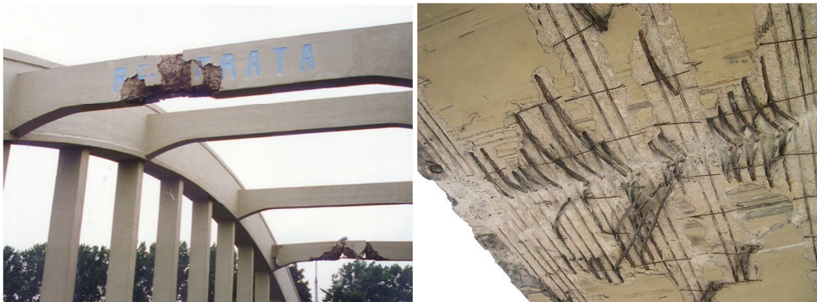
9. Deformations, losses, and loss of material continuity in the elements of the reinforced concrete bridge structure as a result of overloads caused by impacts of vehicles with oversize dimensions
