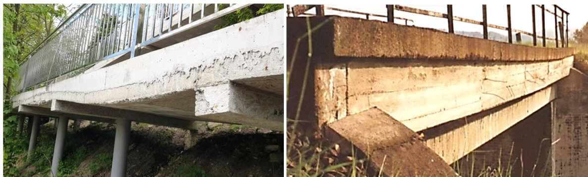
10. Deformations in the form of: incorrect structure geometry (on the left) and changes in the geometry of the element axis - permanent deflection of the span structure (on the right)
