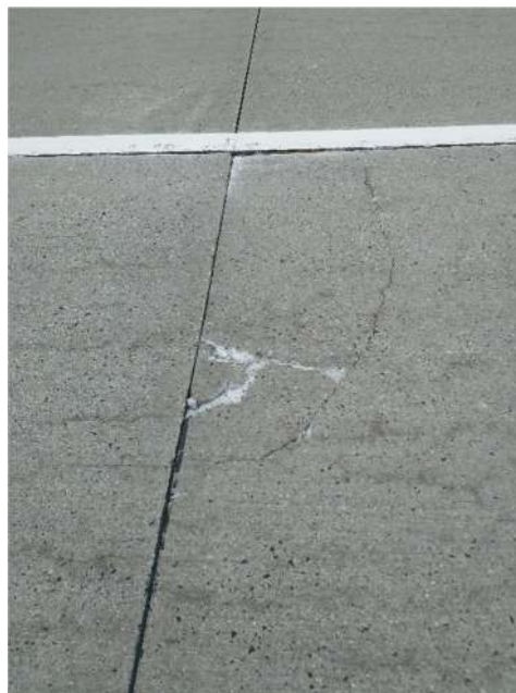
1. Plate edge breakage as a result of subsidence
