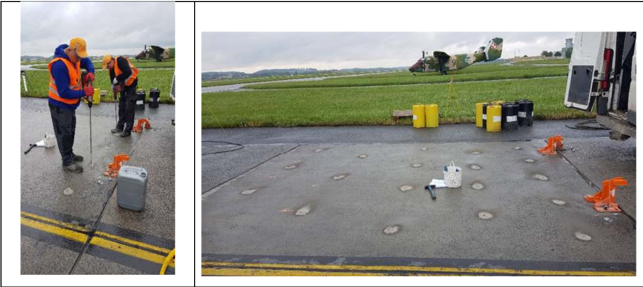
6. Drilling injection holes with a diameter of 14-16 mm (according to the marked grid)
