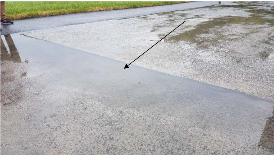
5. View of the plate edge lowering at the parking stand (flooded with water) - slot marked no.2
