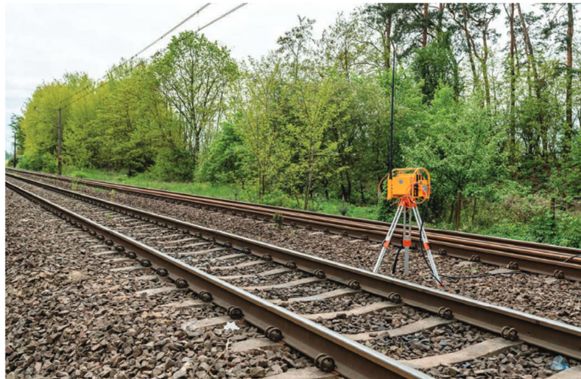
3. A radio transmitter connected to an inductive wheel detector of a rail vehicle
