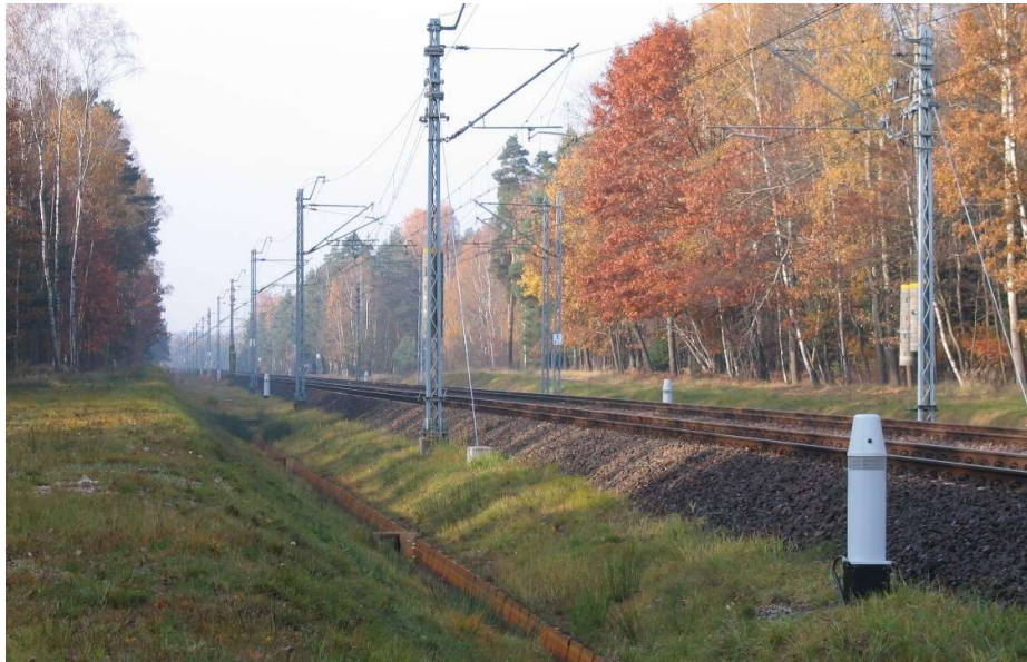
1. Animal Protection Equipment UOZ-1 on the E30 line, section Węgliniec – Bielawa Dolna source: NEEL
