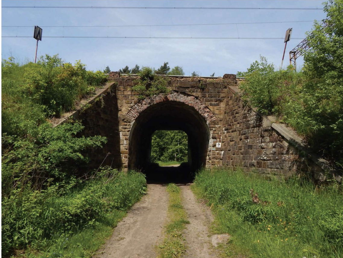
1. An object not properly secured against falling from a height
